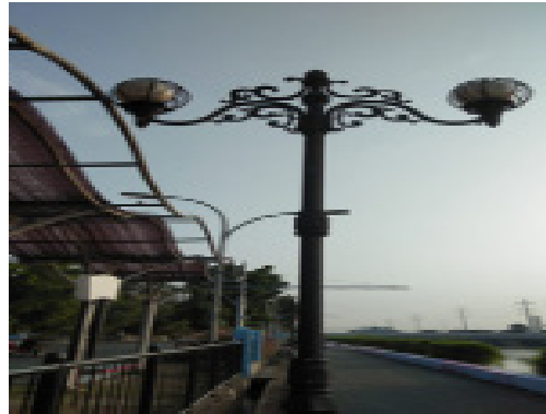
Park Light Not Working
